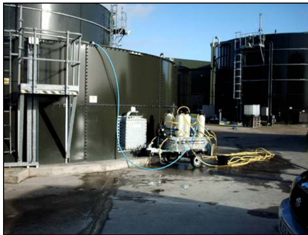
Figure 24. The pilot rig at JE Hartleys
