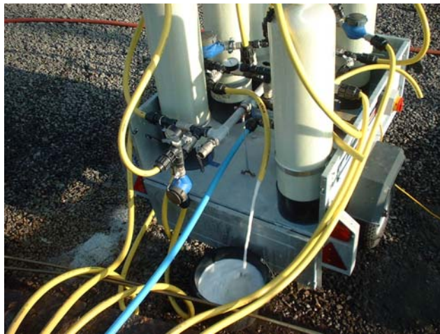
Figure 18. Backwashing filter 4 to the backwash storage vessel.
